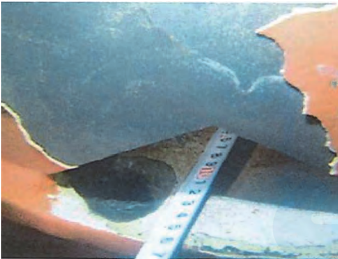
Fig. 4 Corrosion around welded parts between distance piece and bluff body
