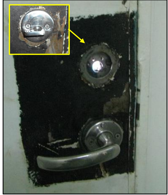
Detached key of fire door
