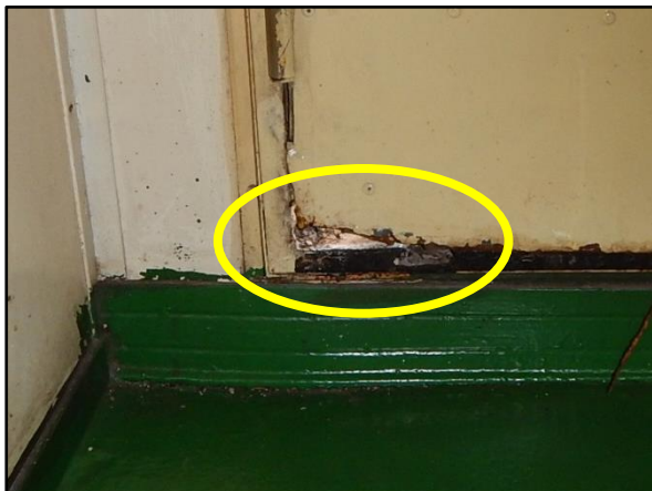
Wasted fire door
