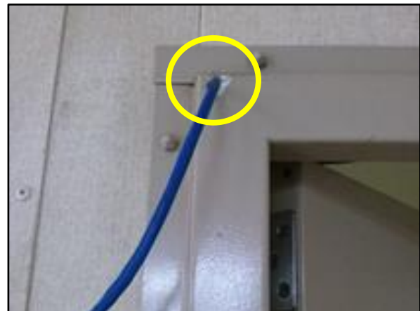
Inappropriate cable penetration
