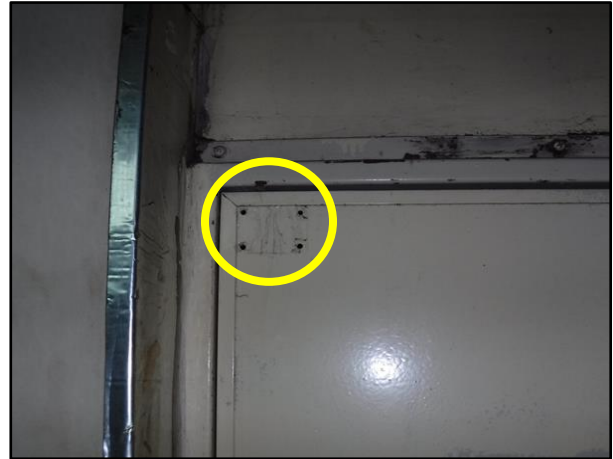
Inappropriate fire door repair
