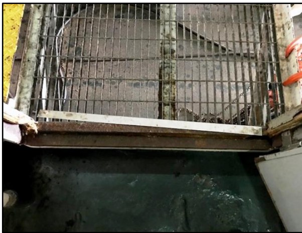
Detached fire door frame
