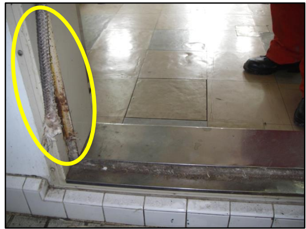
Detached fire door packing
