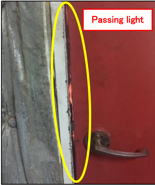
Gap between fire door and frame
