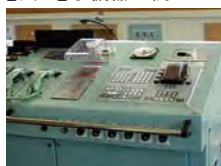
(主機の制御・警報盤)
