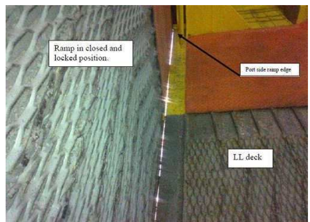
Stern door in closed position: no weather tight due to possible deformation.
