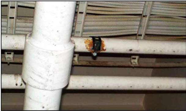
Temporary repair on piping without reporting to PSC
