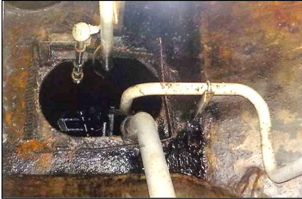
Dirty condition in engine room
