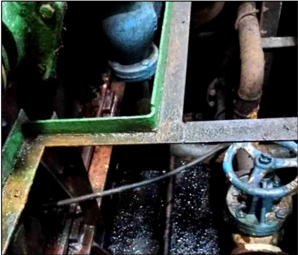
Dirty condition in engine room
