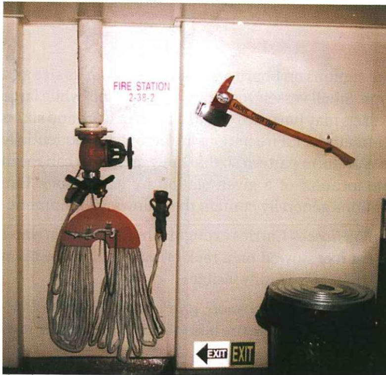
Fire hydrant, fire hose and fire nozzle (Referenced from Marin fire fighting)
